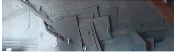
Temporary metal patches
