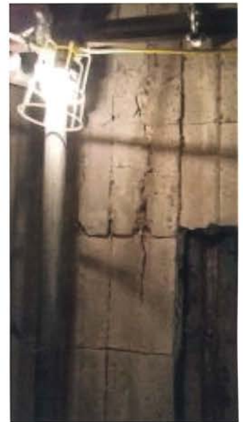
Figure 6: Typical expansion issues in WtE units
