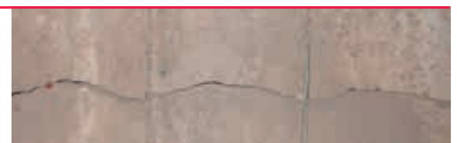
The oxidation of the tiles leads to an expansion and weakening of the structures
