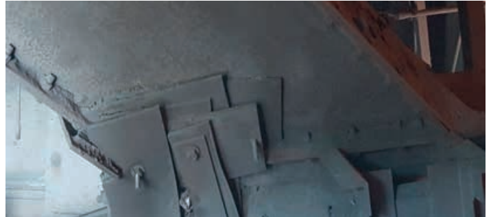
Temporary metal patches
