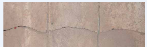
The oxidation of the tiles leads to an expansion and weakening of the structures
